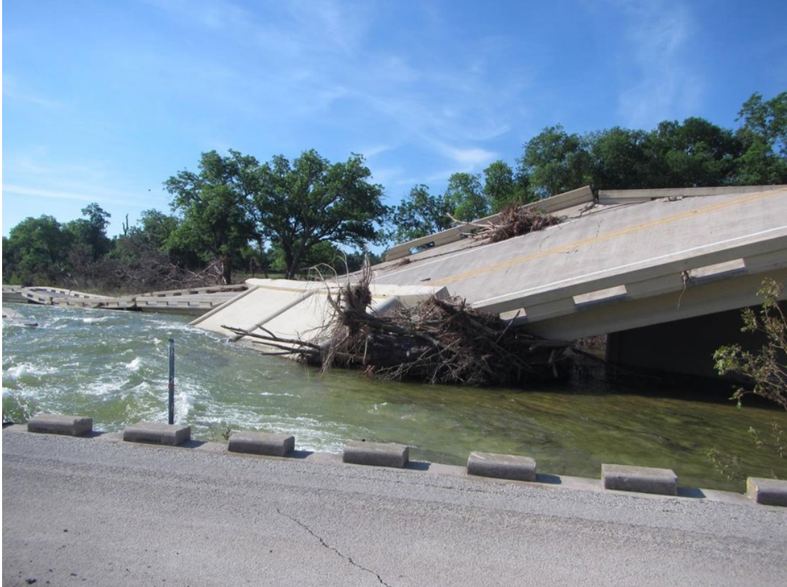
Figure 1-23: Memorial Day Flood Photo
